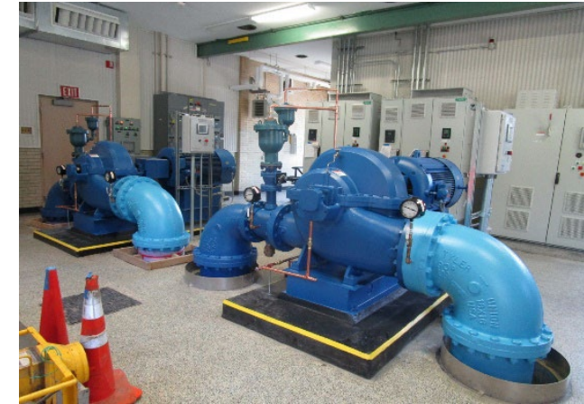
New Pumps at Commonwealth Avenue
